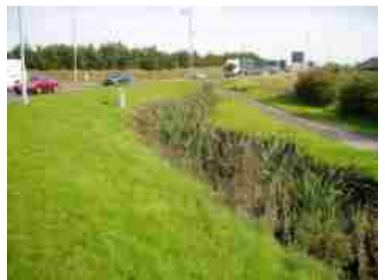
Typical image of swale
